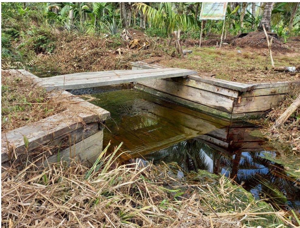
Figure 9. The canal blocking built by the community in Rambaian Village, Indragiri Hilir Regency
